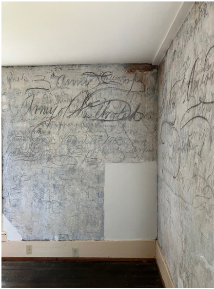
Graffiti covered the walls (Sam Laudenslager)
